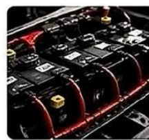
Lithium battery charging and discharging
